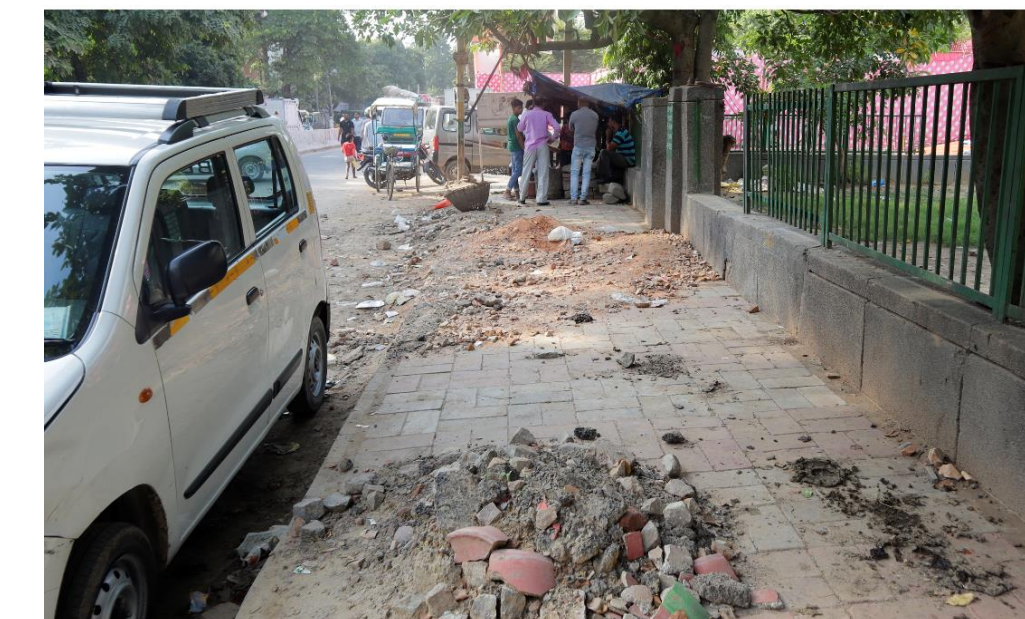
Low maintenance of footpath
