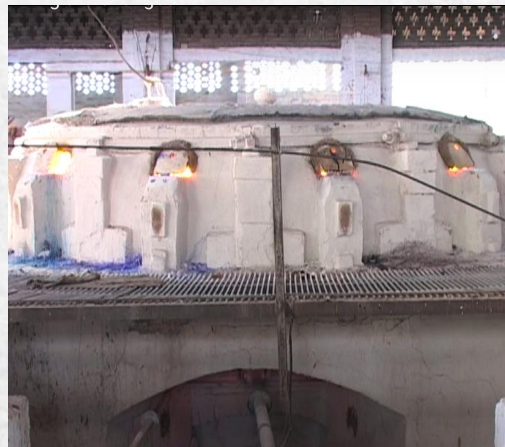
Retrofitted Gas Furnace
