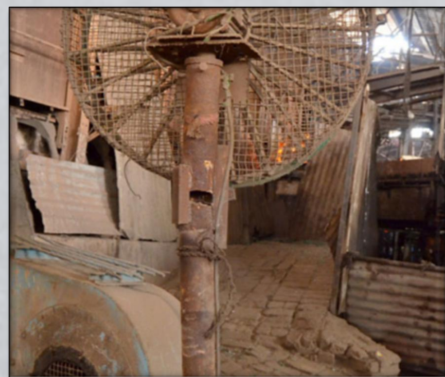
Fan for reducing heat In the factory
