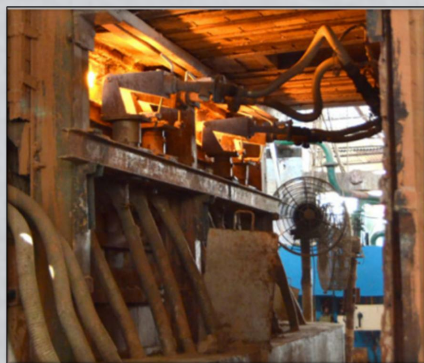
Gas burner of furnace
